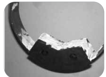
Additional sealant applied to V-Block saddle joint between the two saddle halves. (Chilled water below 50°F).
